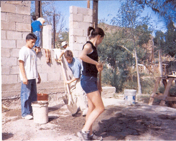
These Seattle teens and mentors journeyed to build a new wing at an orphanage in Guaymas, Mexico
